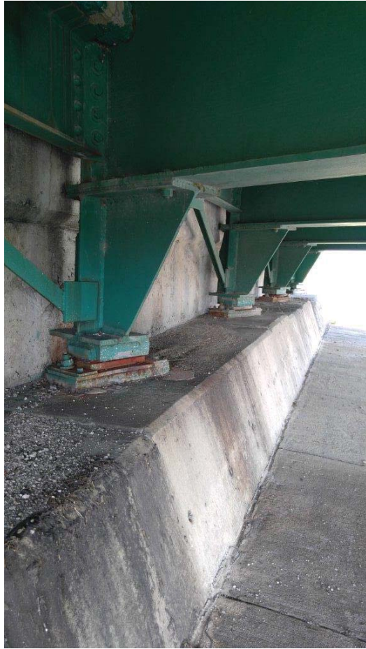
Green Paint under Bridge (LBP Sample #1)
