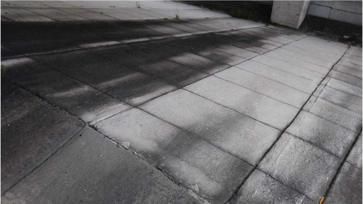
White paint on Caulking under bridge (LBP Sample #5)
